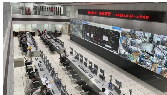
New Jingzhou site central control room
